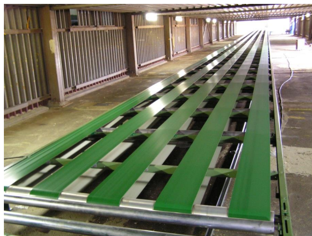
Fig. 1. Conveyor belt system in a PU foam factory
